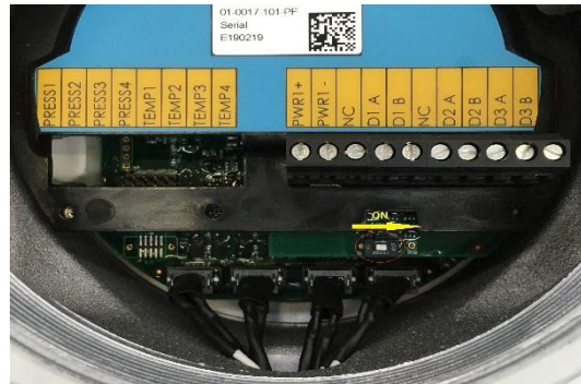
Figure 5-1-3 Line termination resistor switch
